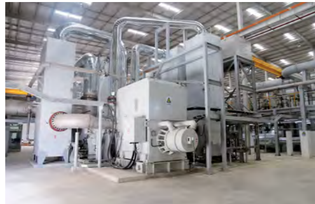
10MW Compressed Air Energy Storage System 10MW 压缩空气储能系统
