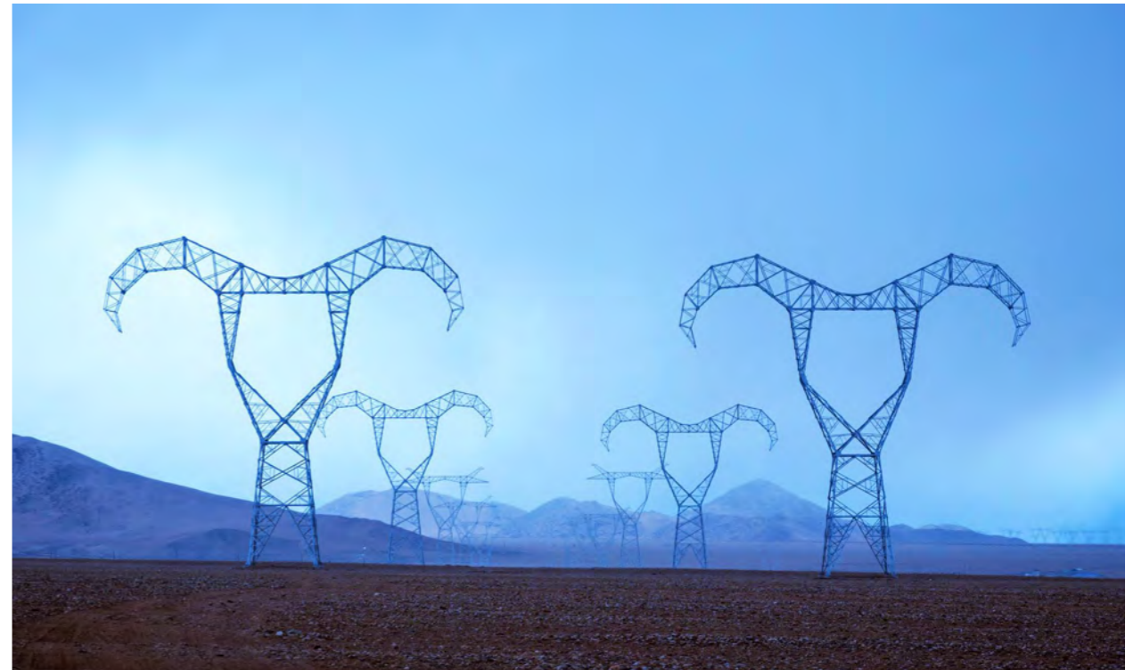
Transmission line towers 输变电塔架
