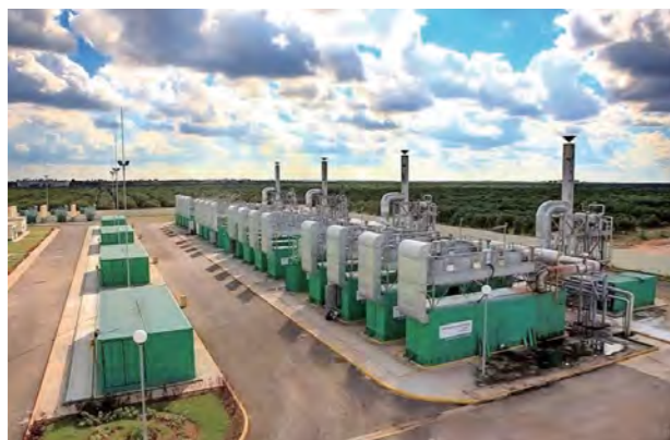
Container Type Heavy Fuel Oil Power Station 集装箱式重油电站
