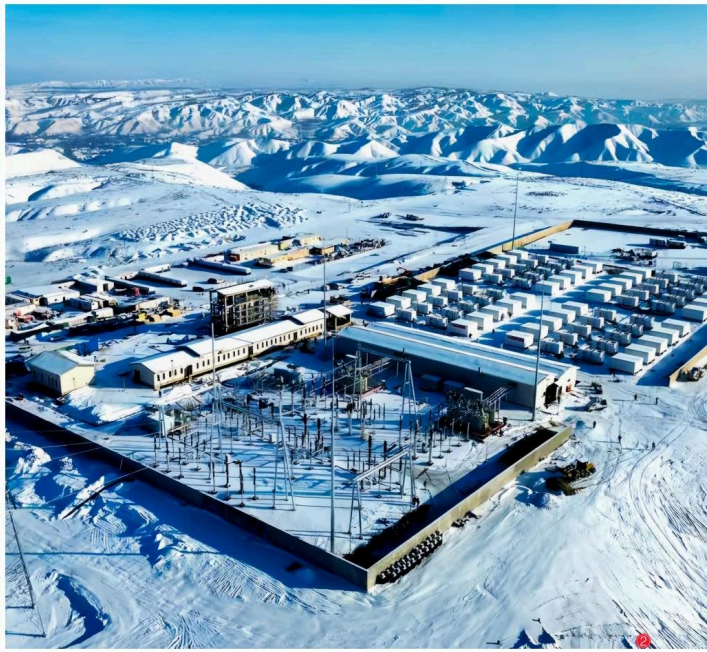
Yingcheng Compressed Air Energy Storage Power Station Demonstration Project in Hubei, China (Principal Investment and Construction)
